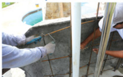
2. 5 Ft Wall sections are wired to rebar frame as back of cave.
